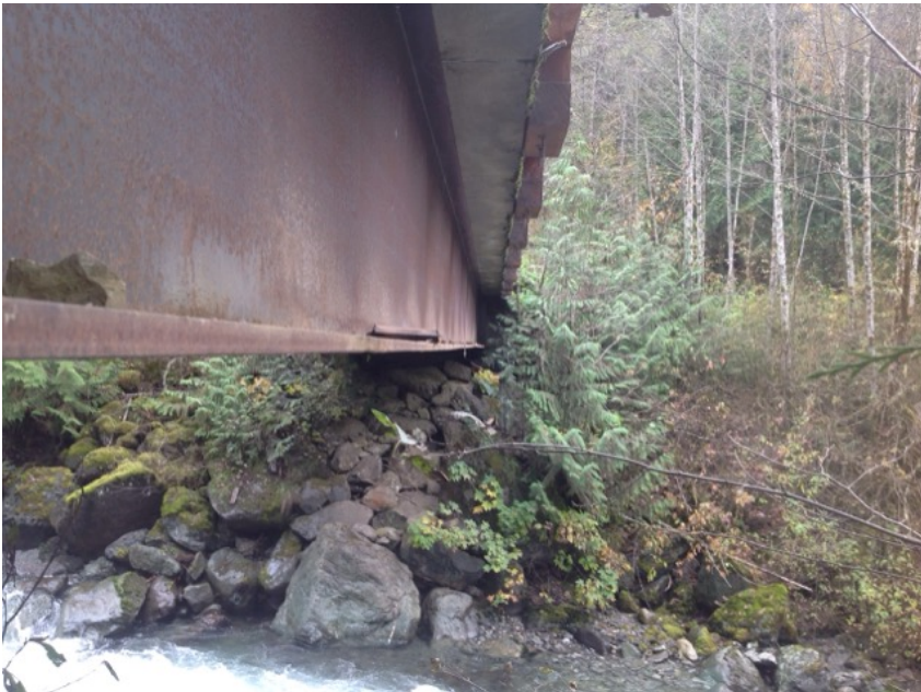
slight undulation of bottom flange - down stream girder
