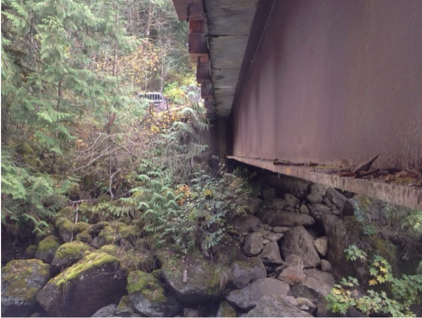
slight undulation of bottom flange - upstream girder
